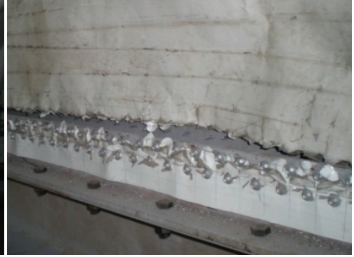
Figure 27 - 10\delta_y ; rear side plate-to-frame connections, lower edge, torn from the screw edges
