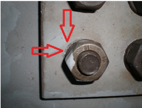
Figure 17 - Crushing of the connection on the web of the beam
