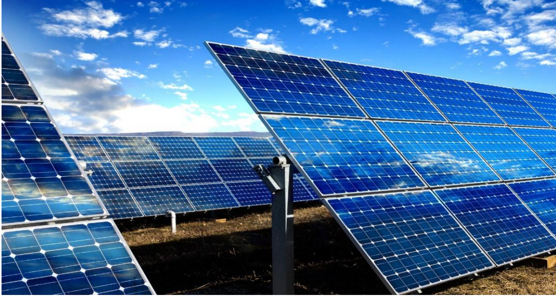
Figure 2.1. Solar panel field.
