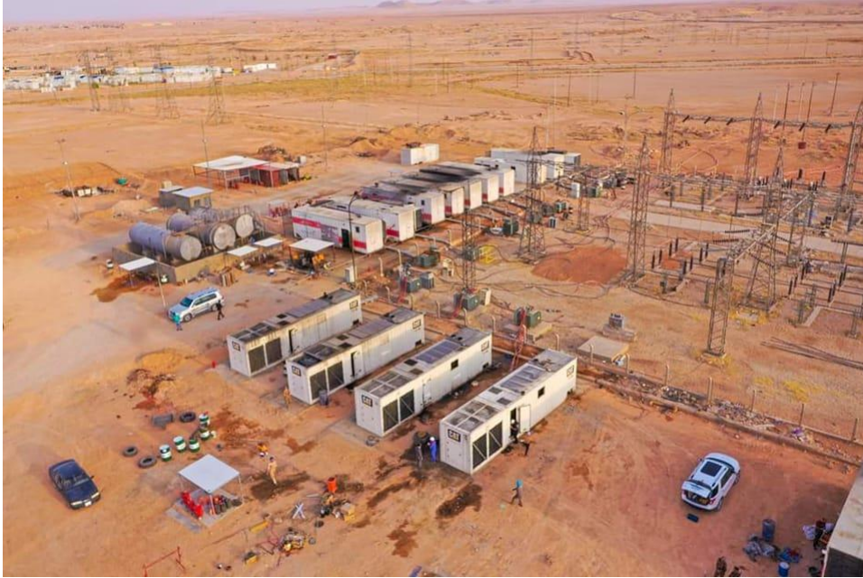
Figure 3.16. The power system plant in Rutba city.
