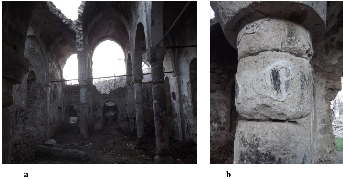
Figure 1. a. An inside view of an abandoned church, b. Detail from a column of which the lead in between the pieces has been snatched-off.
