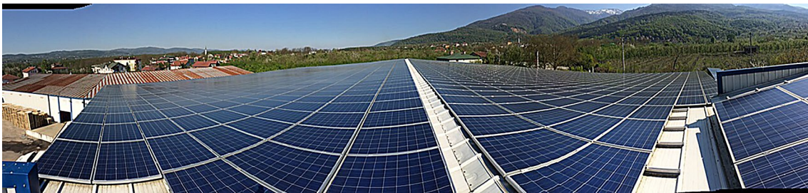
Fig. 1 290.4 kWp grid-connected PV system
