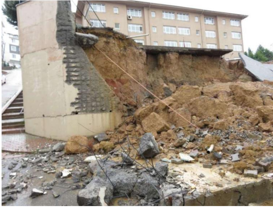
Figure 2.8. Collapsed example of retaining wall in Sancaktepe (url1, 2018; Sönmez, 2023)
