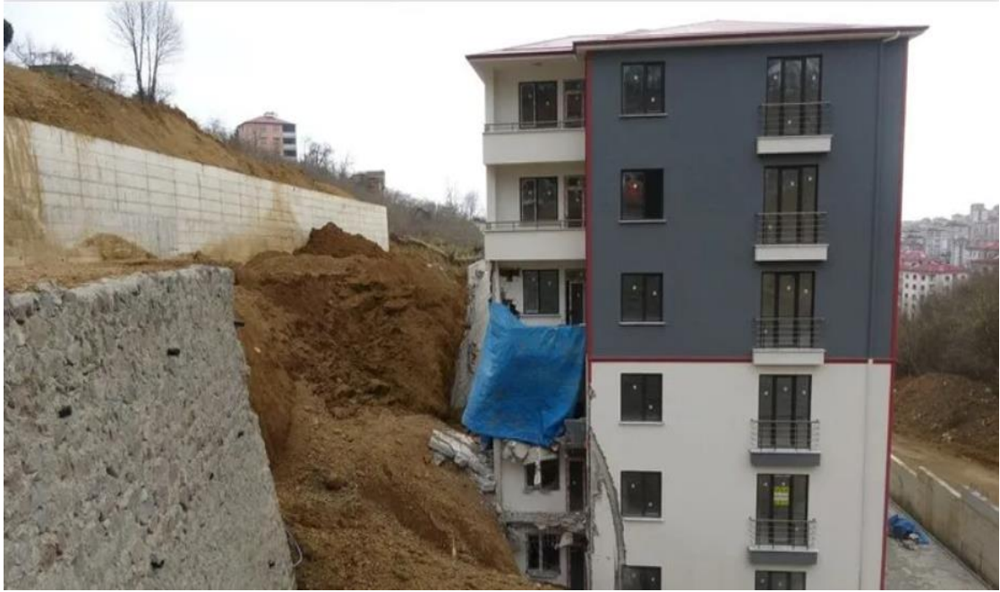
Figure 2.10. Collapsed example of retaining wall in Trabzon (url3, 2022; Sönmez, 2023).
